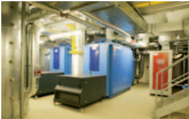
Decentral CHP plant in the cellar of an apartment house
