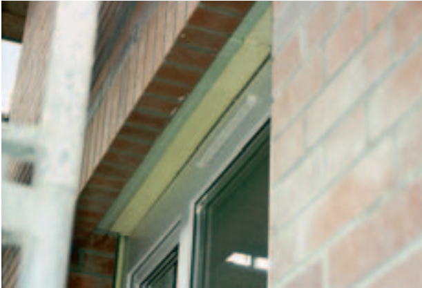
Insulation around a window
