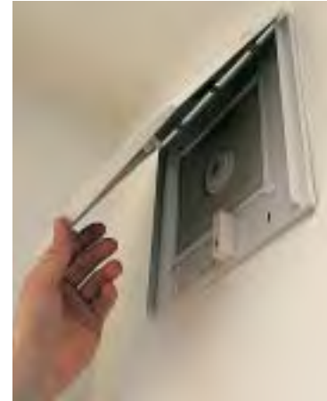
Abluftventilator / extractor fan
